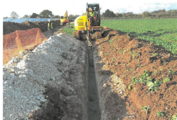
Cable trenching, showing topsoil stripped and set to one side, with subsoil placed on the other side ready for reinstatement (photo courtesy of British Solar Renewables)
