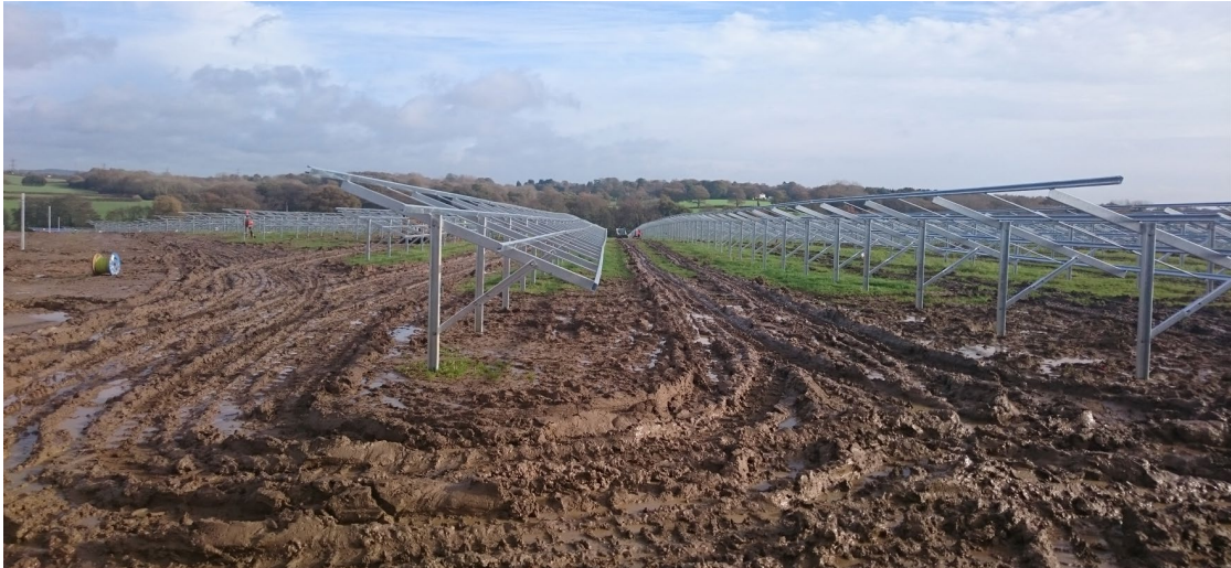
Inserts 36 and 37: Winter Installation (2015) and Operational Site (2022)
